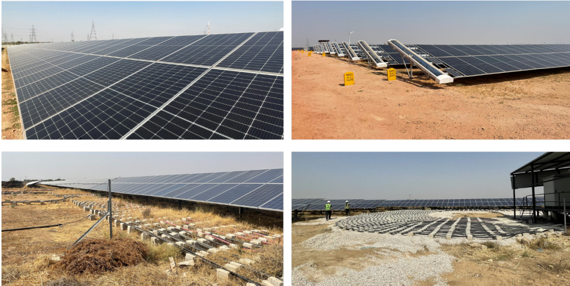
Photo 3: The top two photos represent solar fields with buried cables and well-groomed grounds. The bottom two photos represent solar fields with above ground cables and unkempt grounds, which can increase the potential for hazards.
